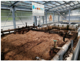
Wastewater treatment tank (aeration)
